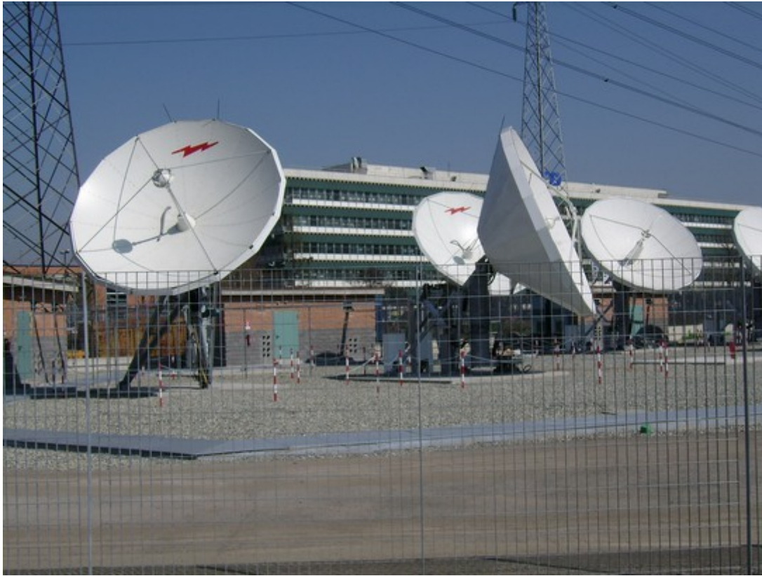
Figure 11: Example of antennas in a teleport
